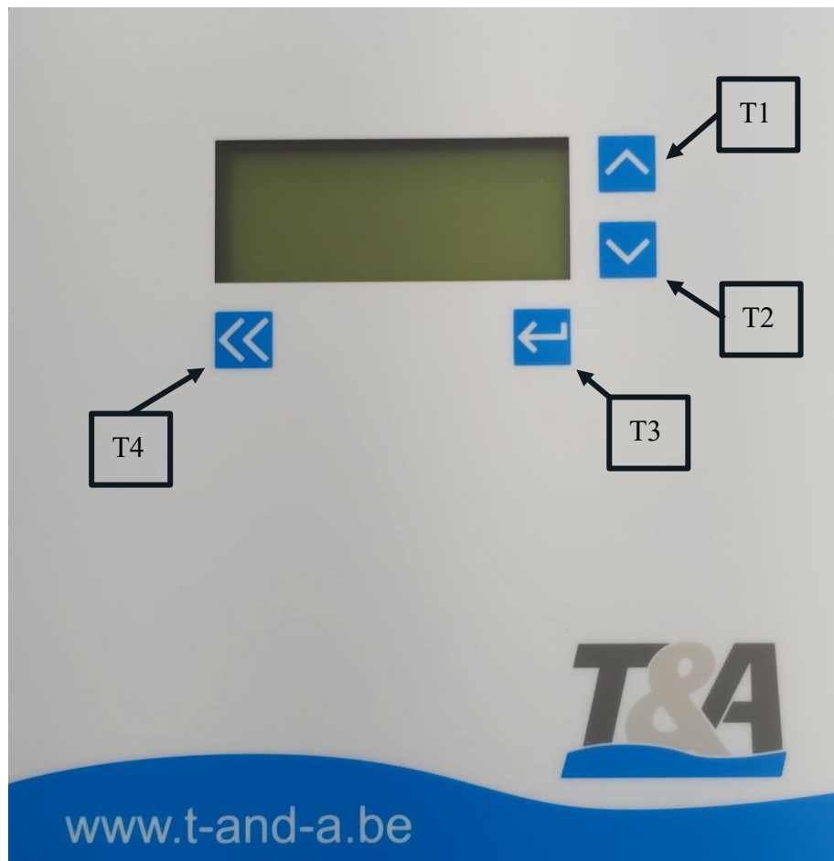
Figure 10 - Front of the control box
